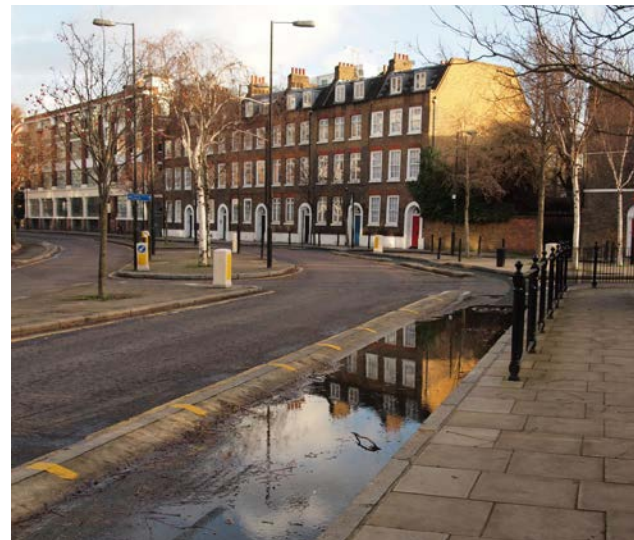
Problems caused by ponding
