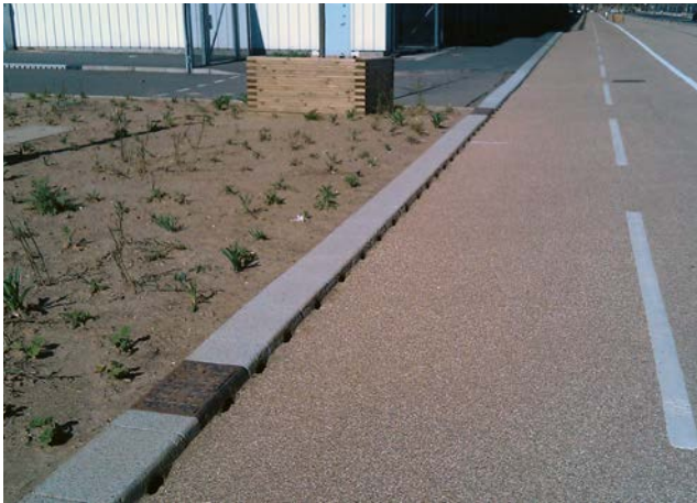
Perforated kerb gullies, as used in a cycle track
