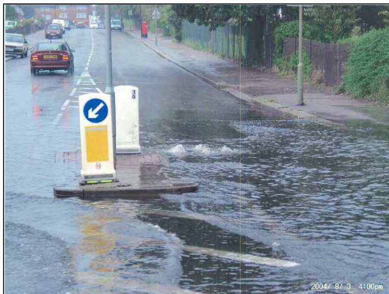
Figure 10 - Photographic evidence of sewer flooding on roads, Colindale, 2004 (courtesy of LB of Barnet Highways Department)
