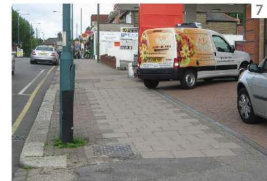
Poor quality, uneven paving
